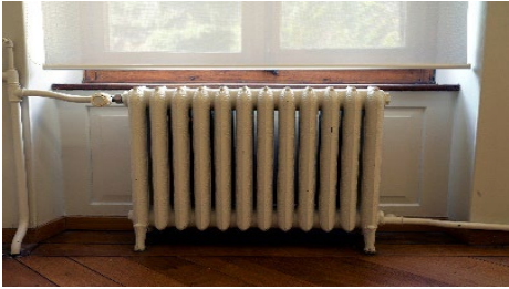
Heating, Ventilation, and Air Conditioning (HVAC)
