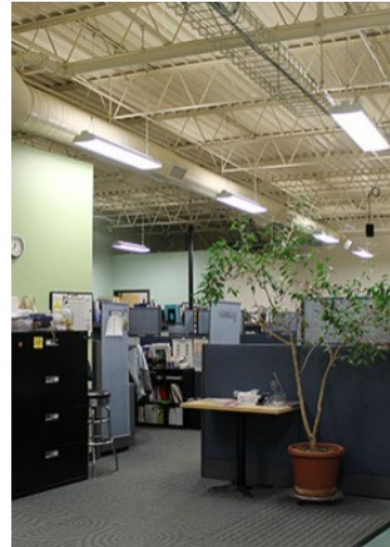
Energy-efficient fixtures in office area.
